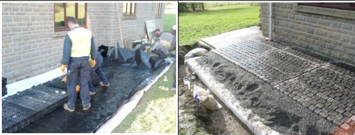
Installation of a rainwater harvester system below a permeable concrete block surface
